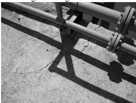
Figura 6. Losa 16 fisura diagonal
