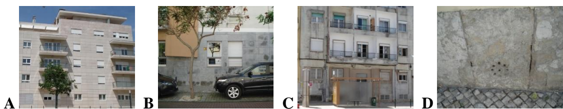
Figure 1. Degradation conditions for stone claddings
