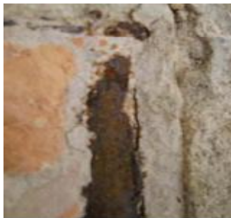
Figure 5. Columns' longitudinal reinforcement eroded (corrosion).
