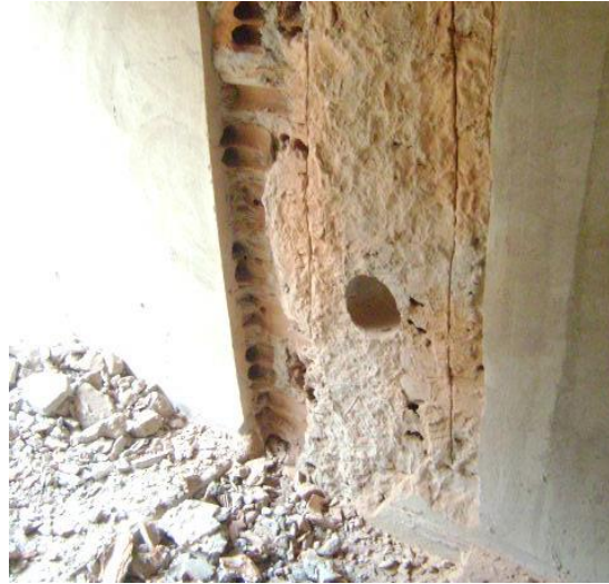
Figure 4. Testimonies' extraction hole in a column.
