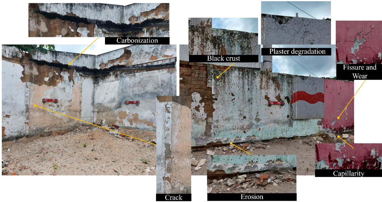
Figure 2. Pathological manifestations observed on the internal walls of the Casarão
