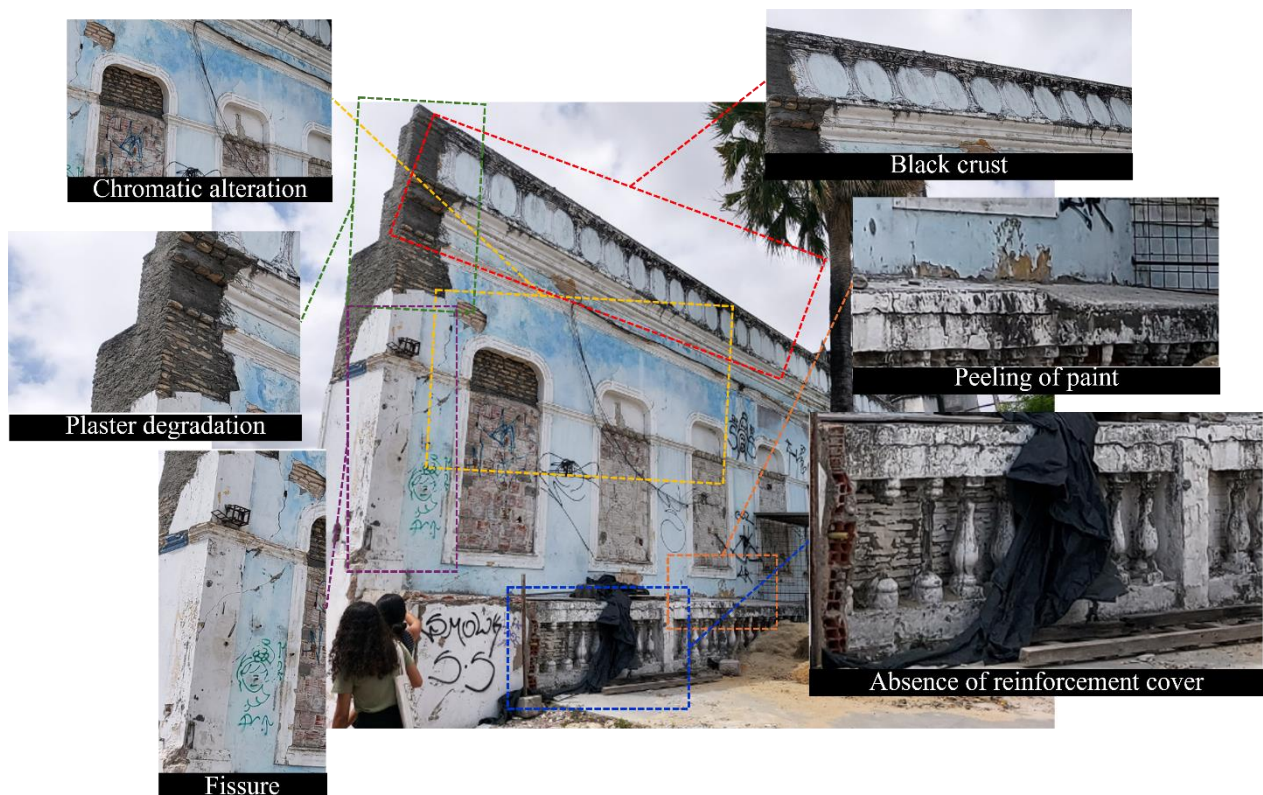
Figure 4. Pathological manifestations identified on the Casarão facades
