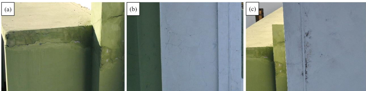
Figure 10. Pathological manifestations on the west facade six months after revitalization: crack, detachments and efflorescence (a), Vesicles and map cracking (b), Dirt and paint stripping (c).
