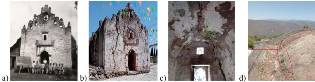
Figure 2. Temple of Santa Catarina; a) preserved building (Biblioteca Tomás Navarro Tomás, 2023); b) current state of the temple; c) and d) Cracks in the keystone and kidneys, respectively. Taken from (Segovia, M. A., 2022).
