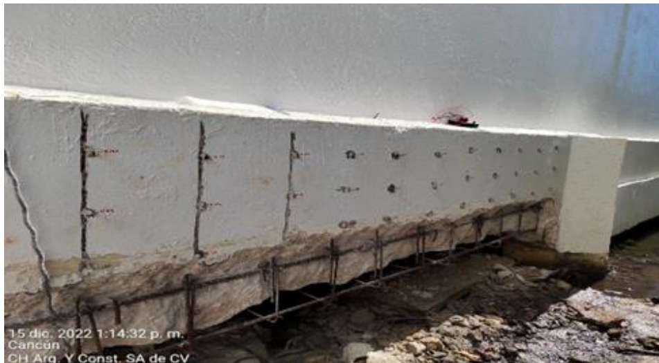
Figure 16. Installation of anodes inside host concrete with installation verification in Cancun, Mexico.
