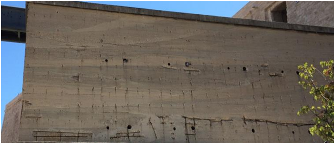
Figure 3. Carbonation-induced corrosion in areas of poor or inadequate concrete cover.
