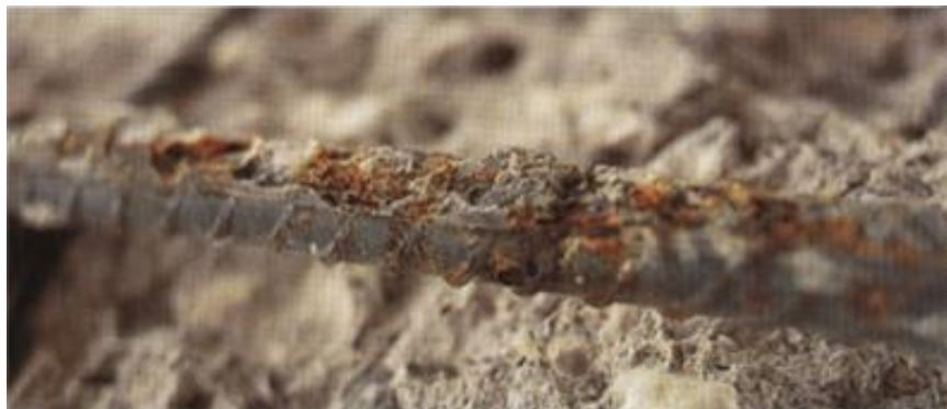
Figure 5. Typical pitting chloride induced corrosion.
