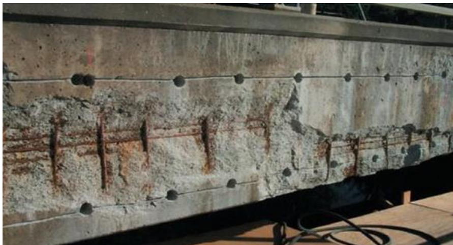
Figure 17. Discrete anodes on a bridge parapet.
