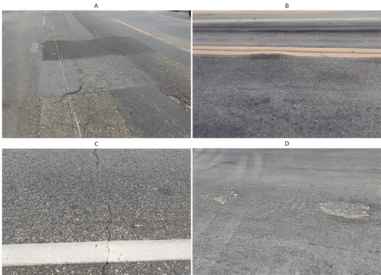
Figure 2. Main distresses found on Highway BR-222: (a) patches and alligator cracks (b) settlements (c) transversal crack (d) potholes and outworning
