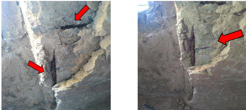
Figure 1. Detachment of concrete and corrosion of reinforcement in element P01
