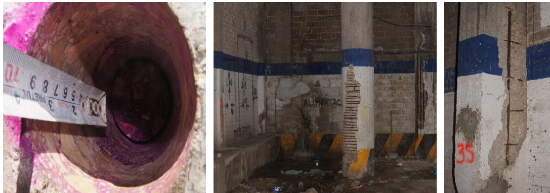
Figure. 3. Carbonation and detachment of concrete.
