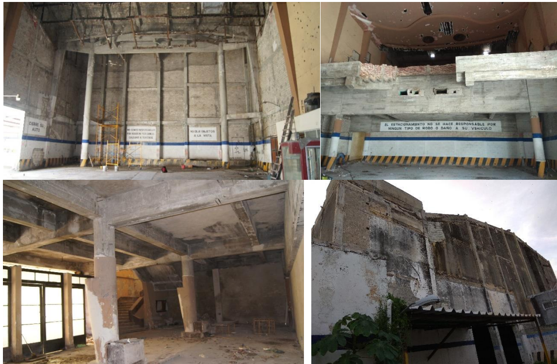
Figure 2. State of the structure before being repaired.
