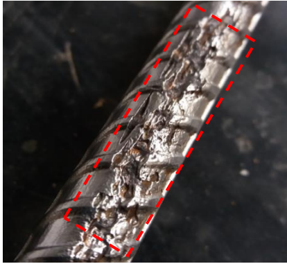
Figure 19. Mass loss from steel bars (L3).
