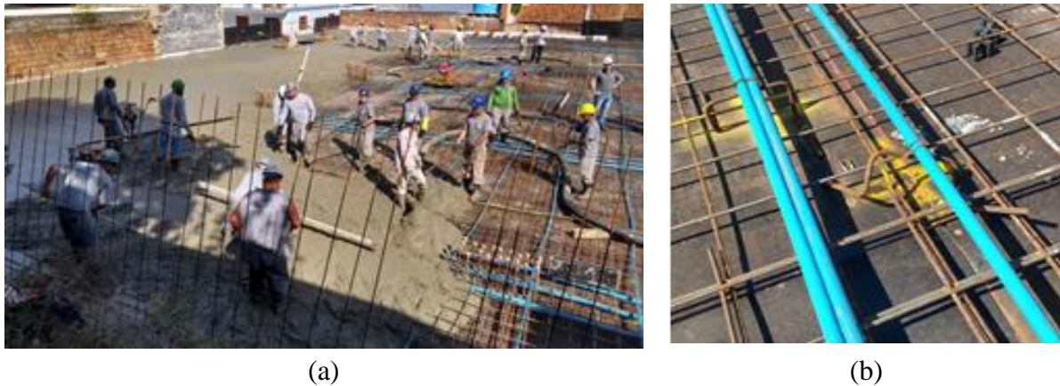
Figure 1. Concrete pouring example: (a) workers in direct contact with the reinforcement and (b) damaged and out of position spacer.
