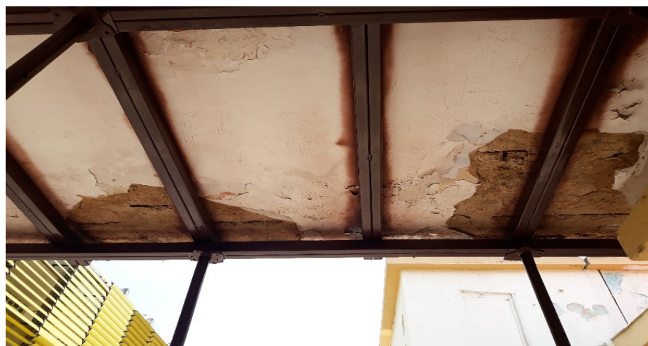
Figure 10. Detachment of concrete at the bottom of the slab
