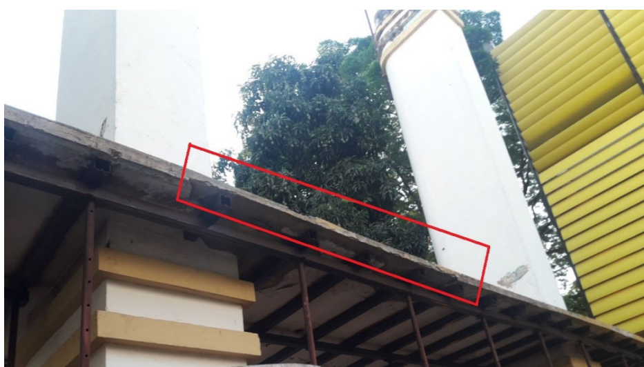
Figure 12. Detachment of the edge of the slab
