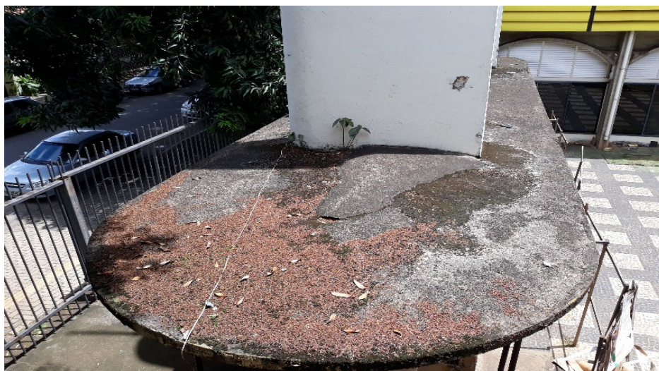
Figure 11. Mold and dirt on the slab
