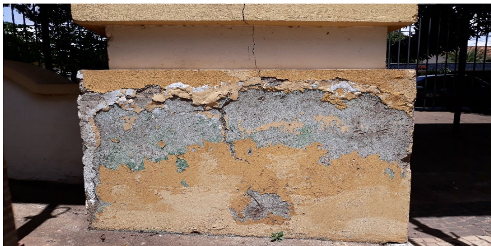
Figure 15: Incidence of cracks and paint discoloration
