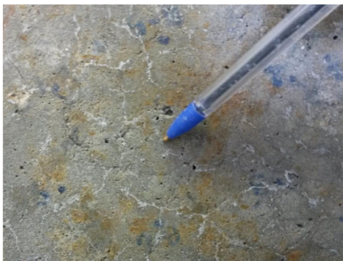
Figure 13. Microcracks in specimens.
