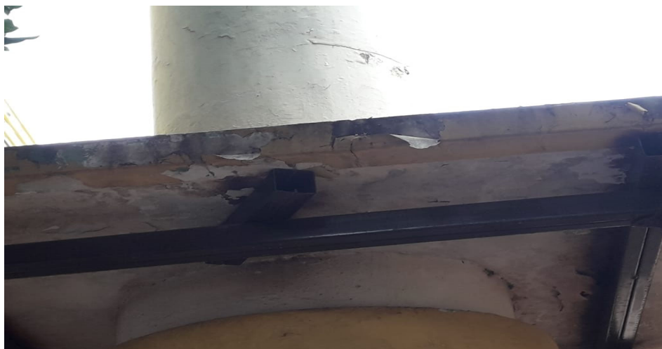
Figure 13. Detachment of the slab paint.
