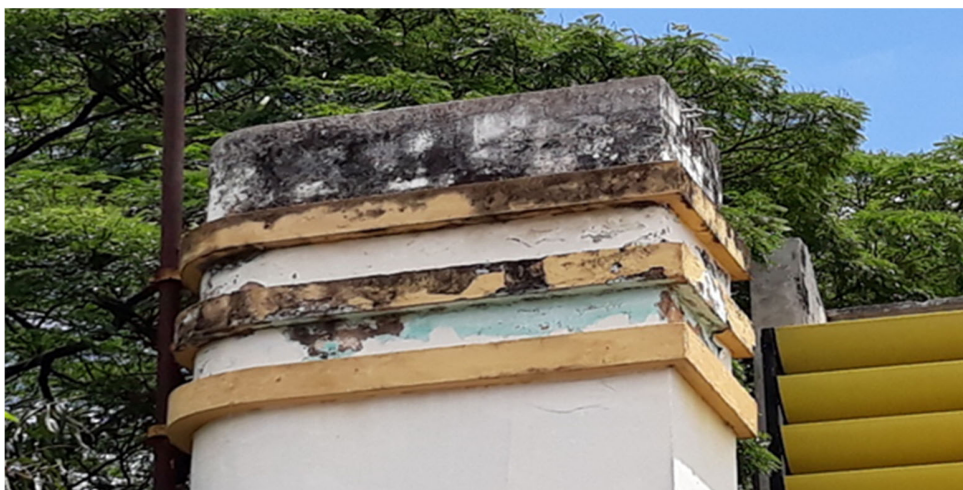
Figure 14. Dirt and detachment of the paint on top of the pillar
