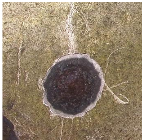
Figure 16. Edge of the corroded area and the area without corrosion (Ribeiro Filho, 2018).
