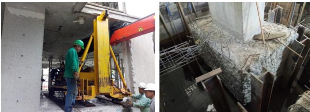
Figure 8. Detail of execution of spiking services (on the left) and of steel piles spiked around the pile cap to be reinforced (on the right).
