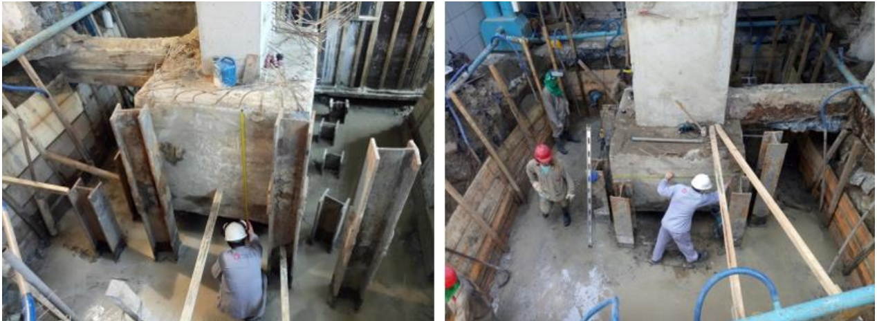
Figure 9. Detail of measurement dimensions of existing pile cap and of the steel piles, after excavation and execution of thin concrete.
