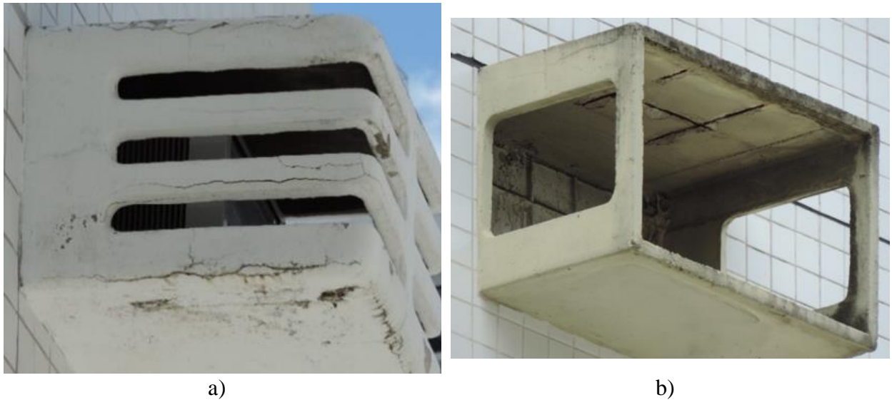
Figure 12. Reinforcement corrosion in window type model: a) fissures; b) concrete detachment.
