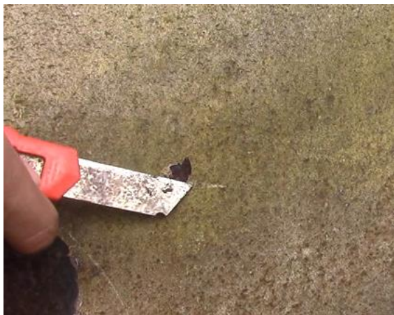
Figure 15. Mechanical damage to the field paint (Ribeiro Filho, 2018).
