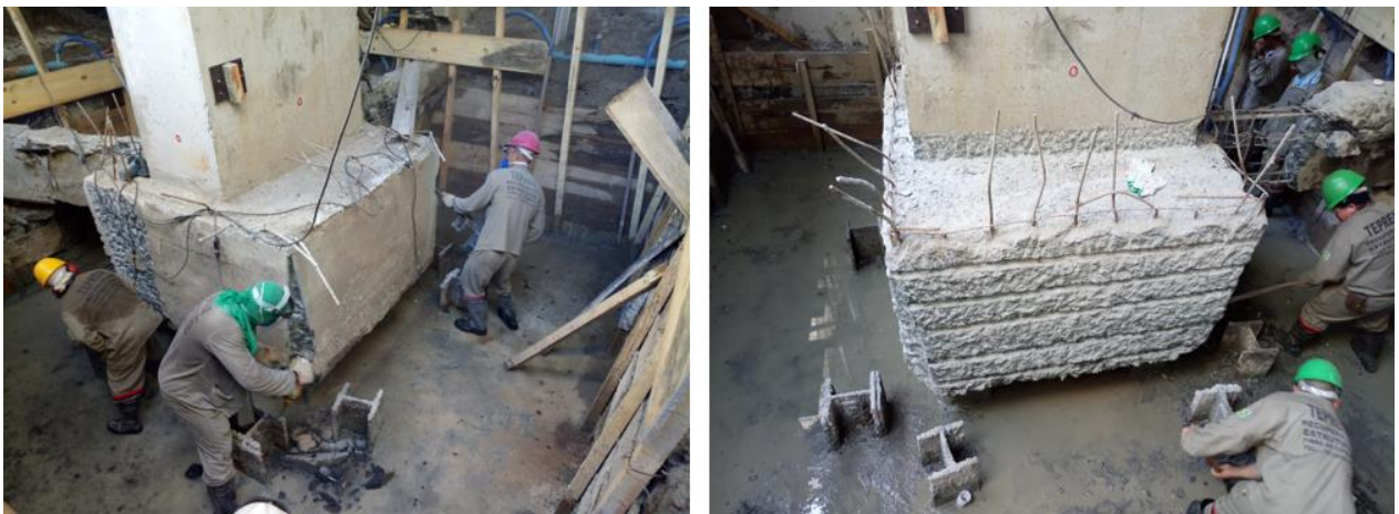
Figure 10. Detail of execution of chamfers and ridges in the edges and lateral surfaces of pile cap.
