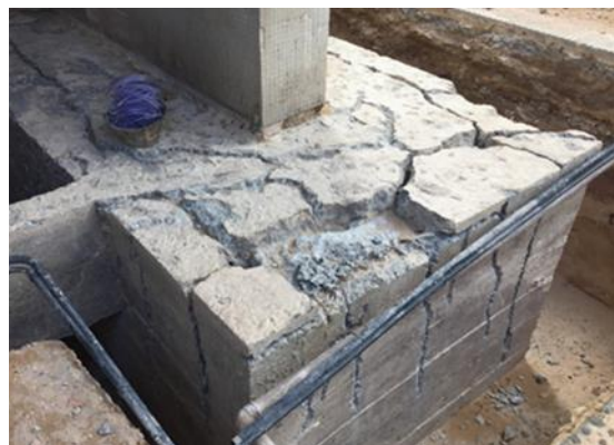
Figure 8. Cracks on a block with AAR.
