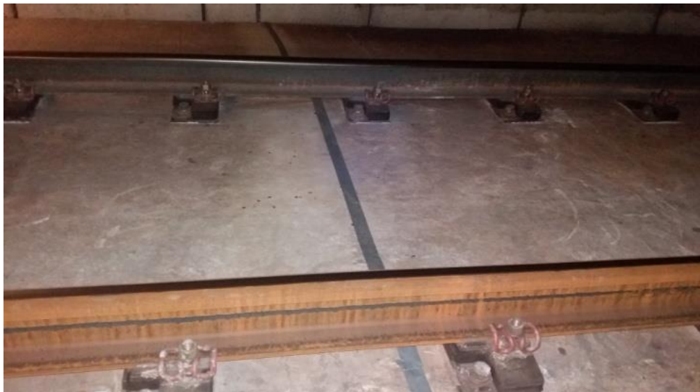
Figure 10. Optical fiber protected under train tracks.
