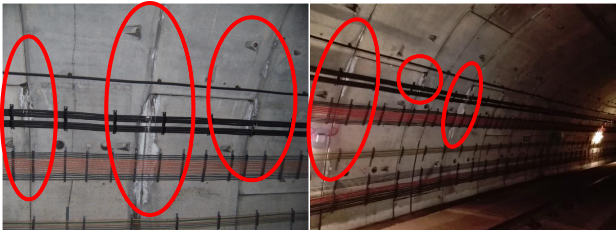
Figure 5. Filtrations (leachings of cement limes).
