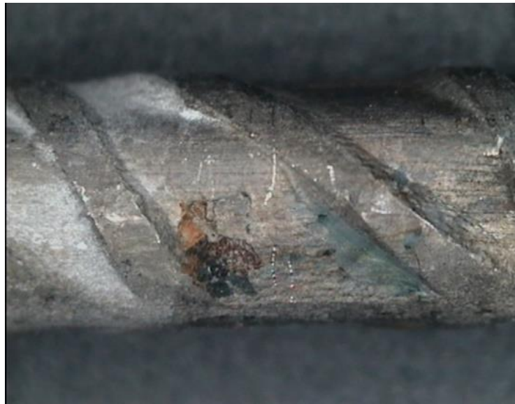
Figure 4. Small spots of corrosion due to chloride attack
