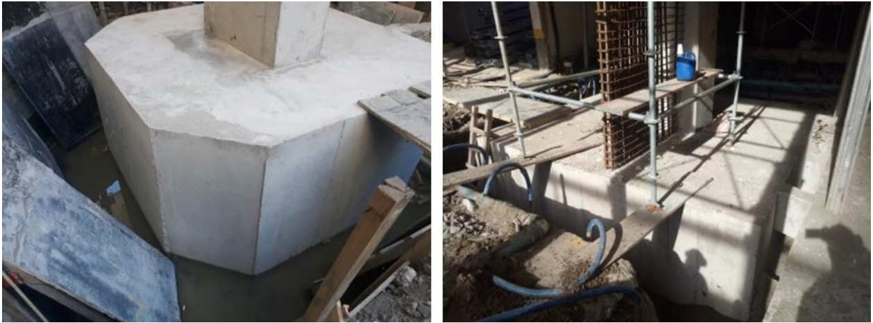
Figure 17. Detail of the visual aspect and the surface finish of concrete of reinforced pile caps.
