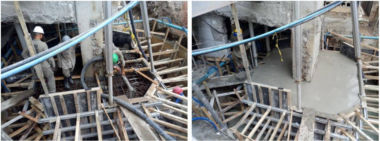
Figure 16. Detail of the concreting of reinforcement of pile cap, made with self-compacting concrete.
