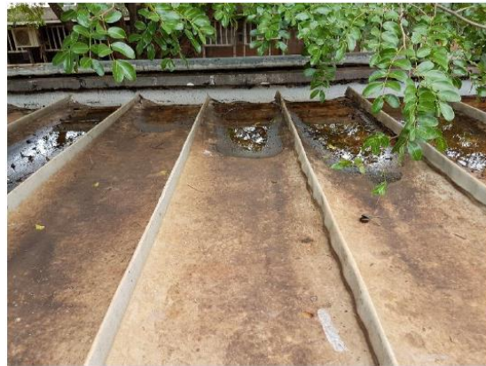
Figure 4. Deformed roof with water accumulation and debris.
