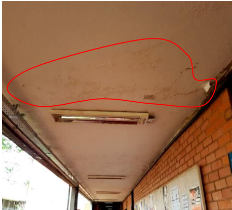
Figure 3. Gutters in the ceiling of the hallway with mold, humidity stains, and peeling of the coating.
