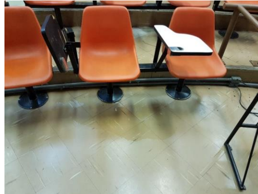
Figure 8. Water puddles formed by dripping
