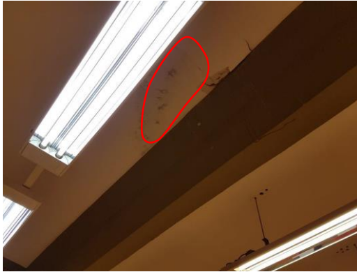
Figure 7. Spotlight humidity on ceiling
