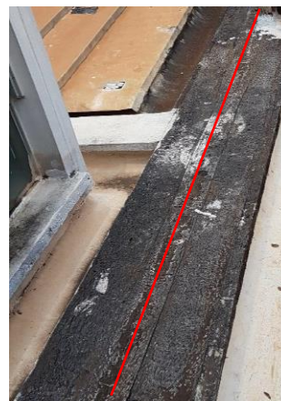
Figure 6. Structural joint without sealant
