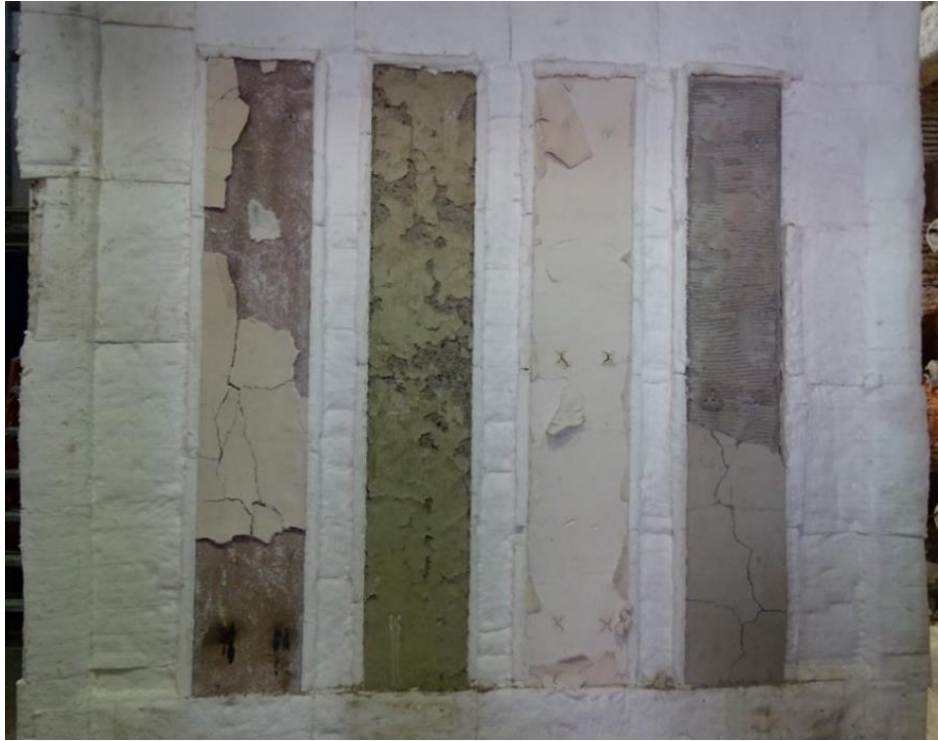
Figure 4. Detail of the elements and coatings condition after furnace opening (event 1): smooth formulated plaster coating, reference element, projected plaster coating and cement-based mortar coating.
