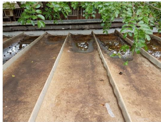
Figure 4. Deformed roof with water accumulation and debris.
