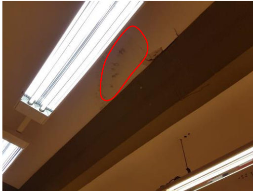
Figure 7. Spotlight humidity on ceiling
