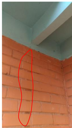
Figure 5. Water dripping on the beam-masonry interface
