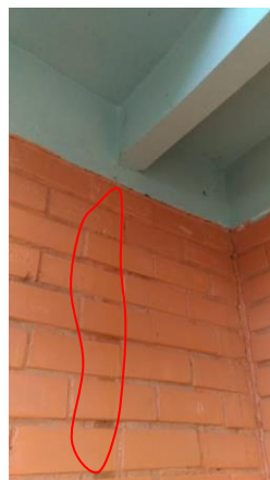
Figure 5. Water dripping on the beam-masonry interface
