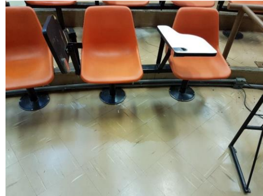
Figure 8. Water puddles formed by dripping
