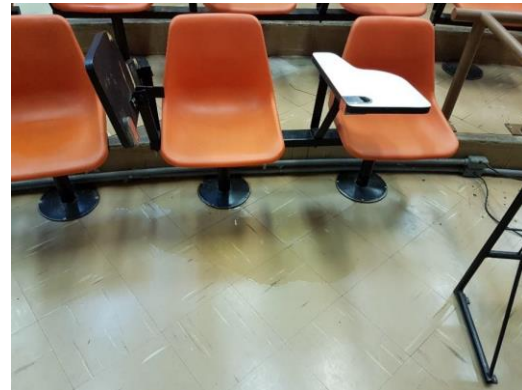
Figure 8. Water puddles formed by dripping
