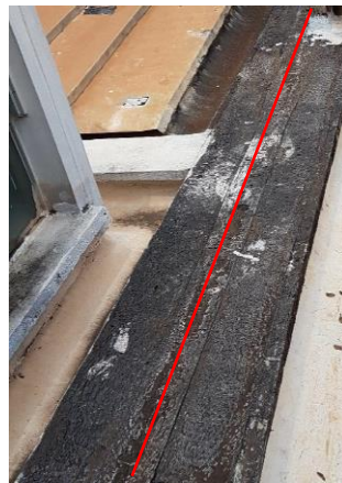
Figure 6. Structural joint without sealant
