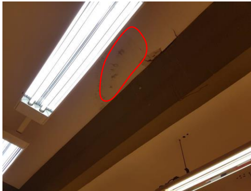
Figure 7. Spotlight humidity on ceiling
