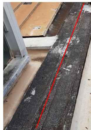
Figure 6. Structural joint without sealant
