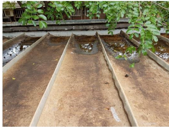
Figure 4. Deformed roof with water accumulation and debris.
