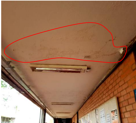
Figure 3. Gutters in the ceiling of the hallway with mold, humidity stains, and peeling of the coating.
