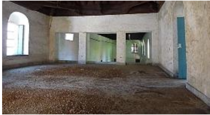
Figure 13. Dirtiness on the walls and in the building because of bat excrement and food remains.
