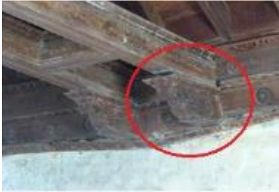
Figure 16. Dropping of corbel under tie rod beam 2 (T2), on axis 2.
