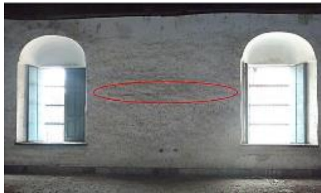
Figure 15. Horizontal cracks in the lower part of the wall (axis 1).
