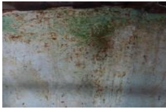
Figure 10. Top wall green patinas in axis 2.
