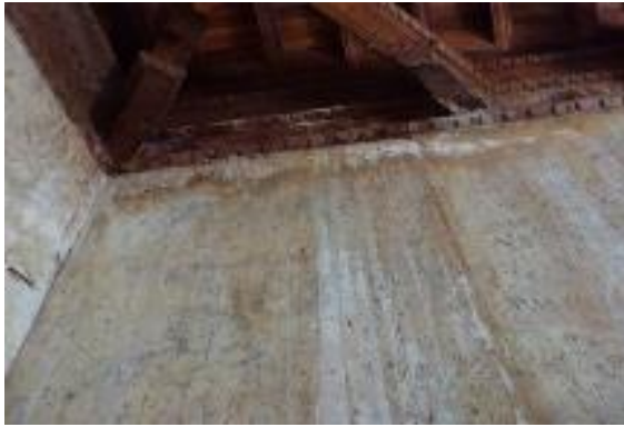
Figure 9. Wall with rain wash in axis A
