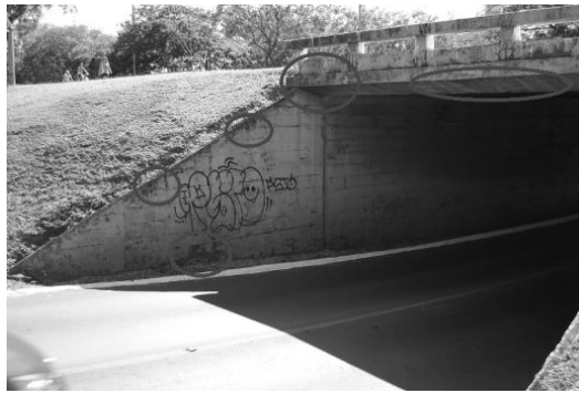
Figure 6. Stains scattered on the structure
