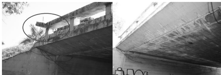
Figure 9. Damage to the bodyguard structure and overview - Damage to the slab due to vehicle tallest than the height of the overpass.
