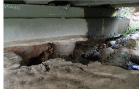
Figure 12. Extreme erosion around the foundation
