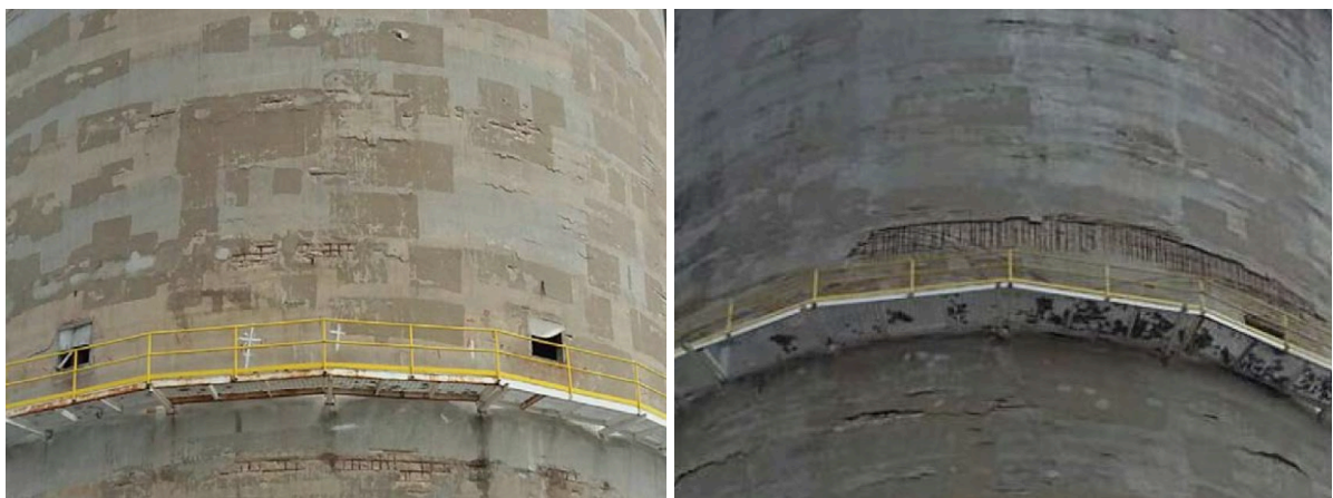
Figure 3. Exposed steel reinforcement, corrosion, concrete spalling and multiple rectangles indicating the sites of previous localized repairs.
