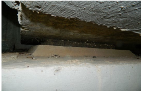
Figure 11. Deformed elastomeric bearing
