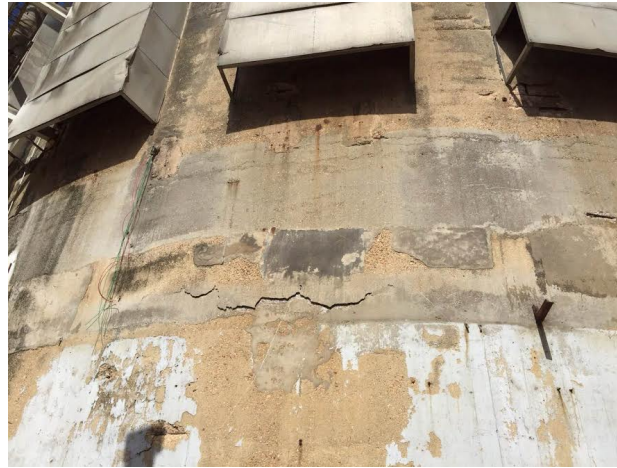
Figure 4. Detail of localized repairs in which the more recent concrete has separated from the original concrete, causing occasional spalling and anodic zones favoring formation of corrosion cells.
