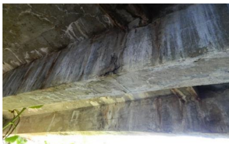
Figure 4. Presence of efflorescence, displacement of concrete coating, and reddish-brown spots due to the corrosion of reinforcement
