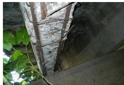
Figure 5. Exposed and rusty reinforcement on beams, some with broken strips
