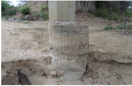
Figure 6. Erosion of the foundation and misalignment of the pillar in relation to the pipe
