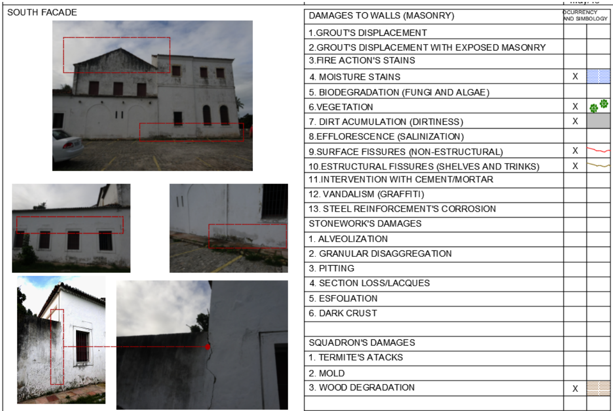
Figure 8. Damage identification form for the south façade of the Carmo Church. Source: Authors.
