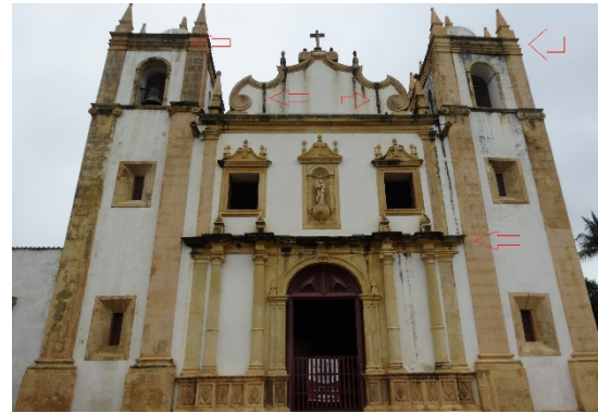
Figure 4. Current damages to the Carmo Church. Source: Authors.
