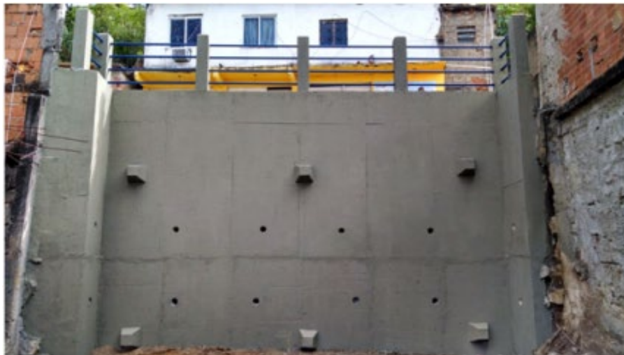
Figure 1. An anchored curtain in a geotechnical hazard area (Author)
