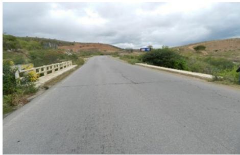
Figure 9. Absence of lateral guard-rail
