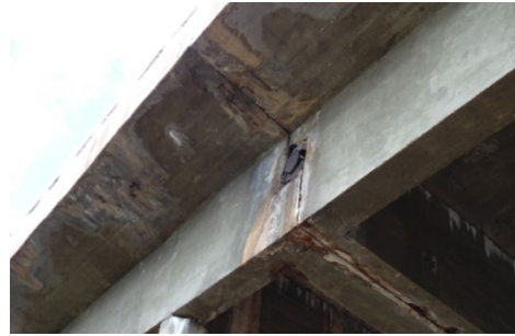
Figure 7. Metal bearing on a Gerber tooth with visible damage and infiltration
