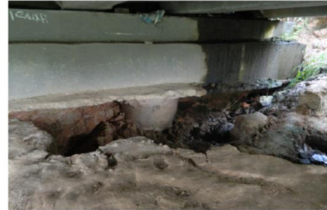
Figure 12. Extreme erosion around the foundation
