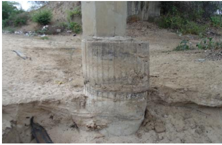
Figure 6. Erosion of the foundation and misalignment of the pillar in relation to the pipe
