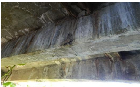
Figure 4. Presence of efflorescence, displacement of concrete coating, and reddish-brown spots due to the corrosion of reinforcement
