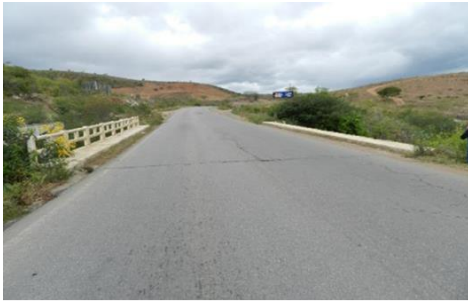
Figure 9. Absence of lateral guard-rail
