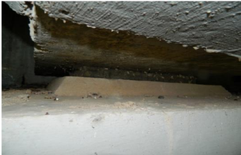
Figure 11. Deformed elastomeric bearing
