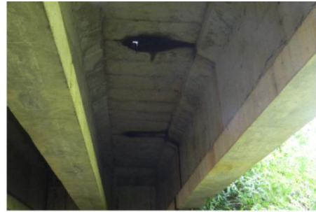
Figure 10. Damaged drain causing infiltration and moisture spots between the beams
