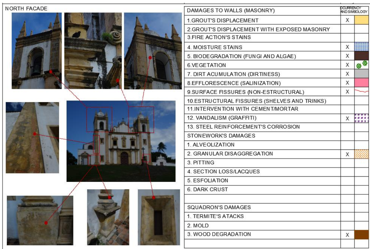
Figure 6. Damage identification form for the north façade of the Carmo Church. Source: Authors.
