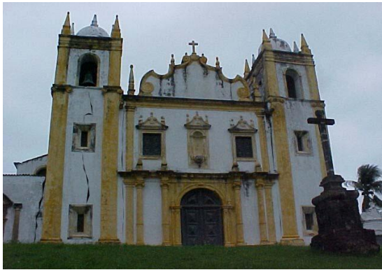
Figure 3. Structural damage to the Carmo Church in the year 2000. Source: Public Collection of Olinda.
