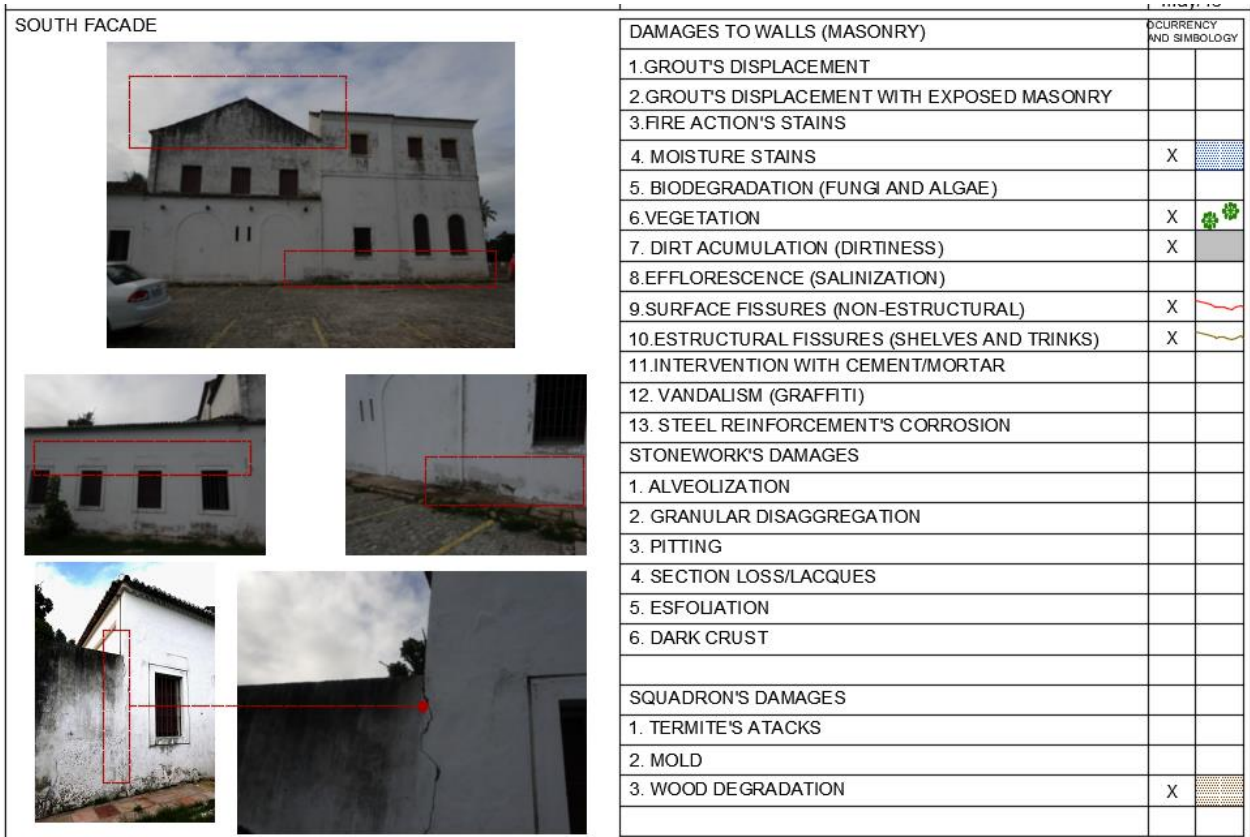
Figure 8. Damage identification form for the south façade of the Carmo Church. Source: Authors.
