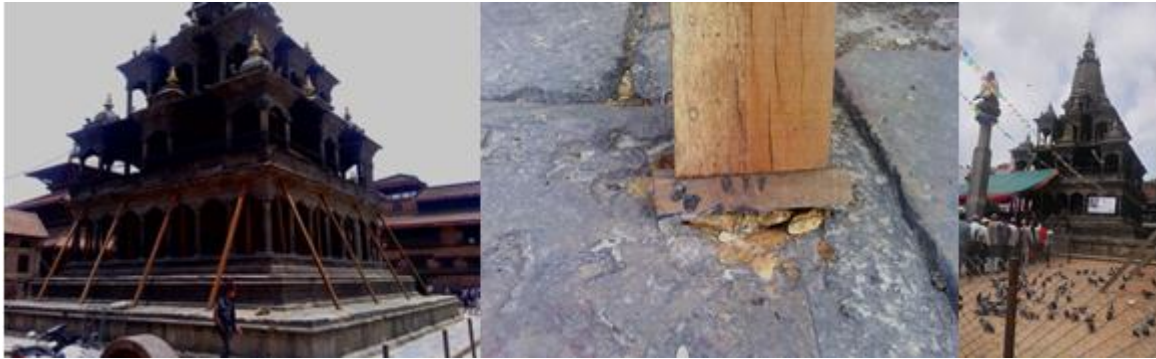
Figure 6. Krishna Mandir at Patan, damaged with post-earthquake protection efforts
