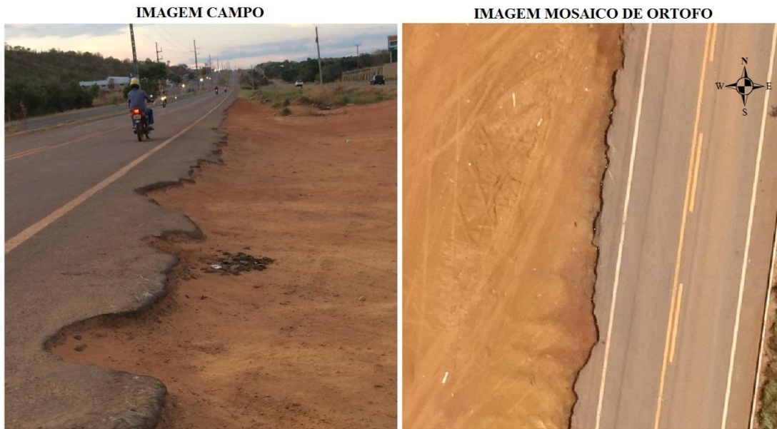
Image 4. Road shoulder pavement loss
