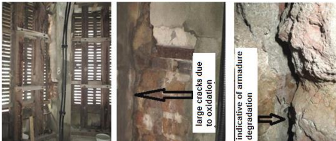
Figures 4 to 6. Fissures caused by the oxidation of the iron clamps inserted in the columns
