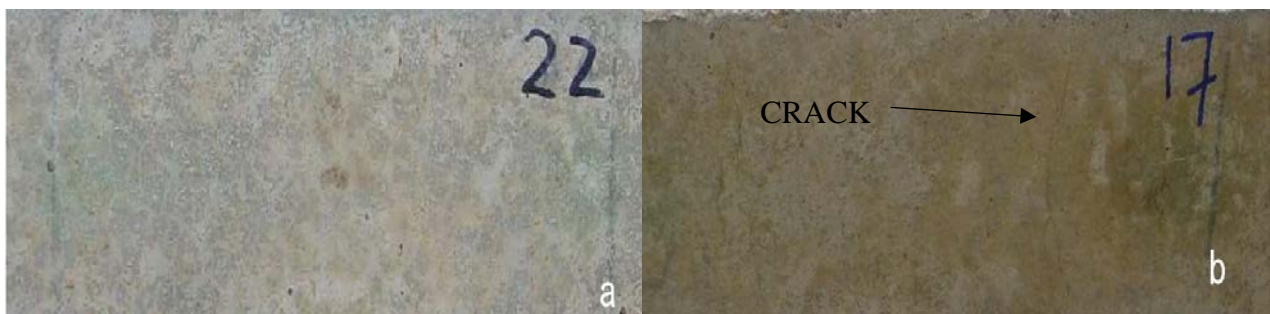
Figure 6. Beams without initial chloride contamination, rinsed with chlorides in the 25-cm central zone (a) non-preloaded (b) preloaded
