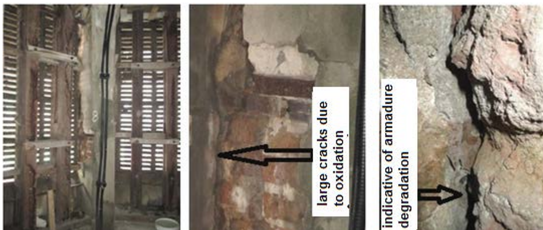
Figures 4 to 6. Fissures caused by the oxidation of the iron clamps inserted in the columns
