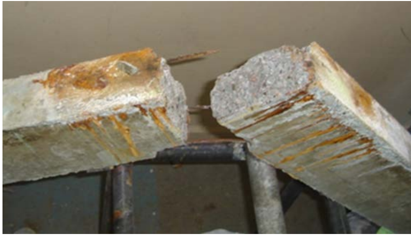
Figure 4. Beam V96 after collapse
